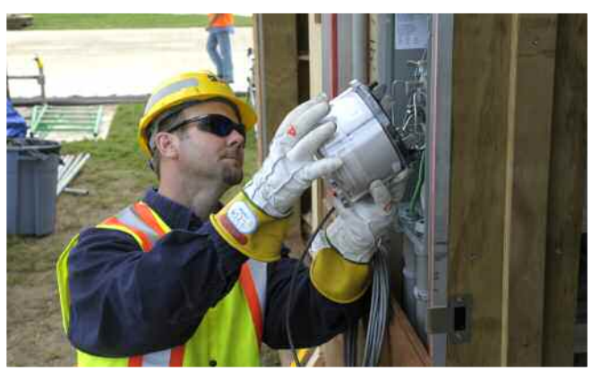
Kenny Kagle, Meter Technician, installs a meter on Team New Zealand's solar house at the 2011 U.S. Department of Energy's Solar Decathlon.
