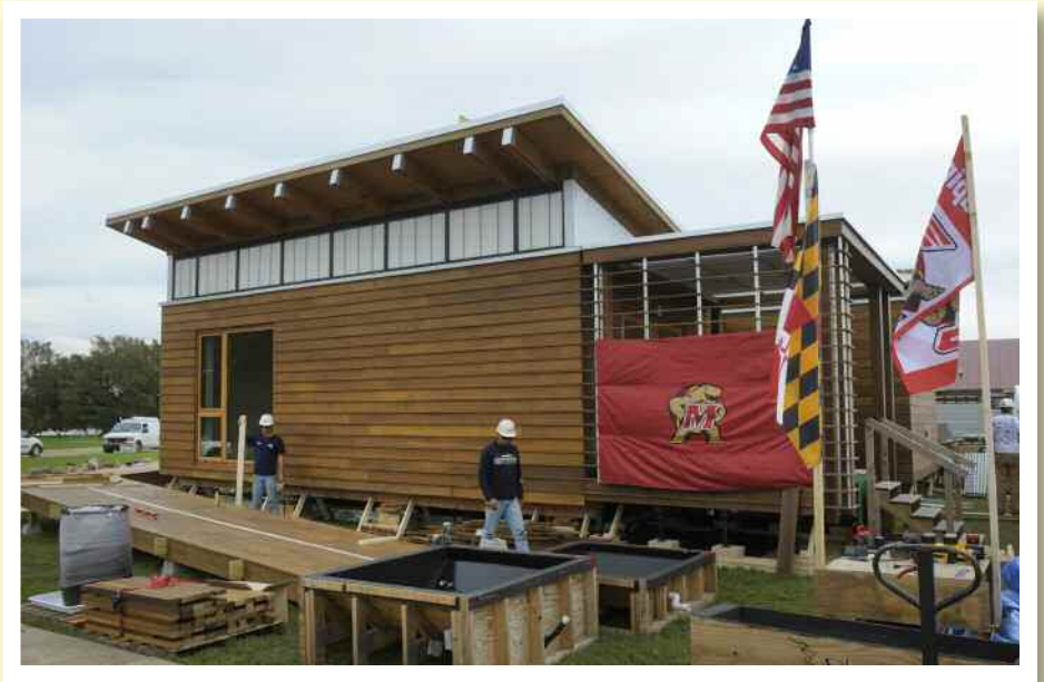
University of Maryland's Solar Decathlon home, under construction, won top honors at the event.
